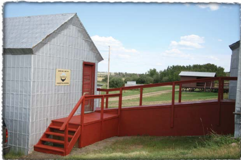
Thanks to the talents of our contractor, Graham Chillingworth, the walkway at the Meeting Creek elevator is virtually complete. The society is now searching for enough specialized tin siding to sheath the lower portion with. It looks excellent and will add greatly to the elevator. Summer, 2007.
